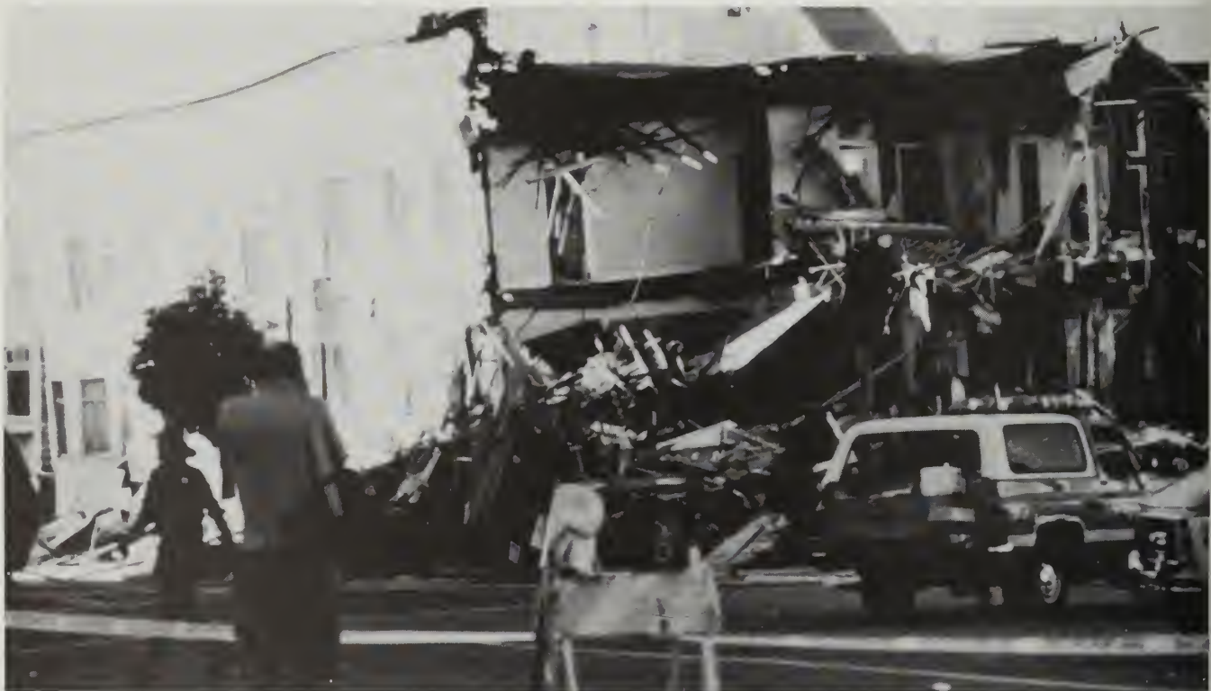
Structural collapse of an apartment complex in San Francisco's Marina District during the 1989 Loma Prieta earthquake. While liquefaction is a hazard in the district, the duration of strong shaking was too short to induce seriously damaging liquefaction. Most damage resulted from enhanced ground shaking triggered by the underlying soft sediments. Photo from Earthquake Engineering Research Institute.
